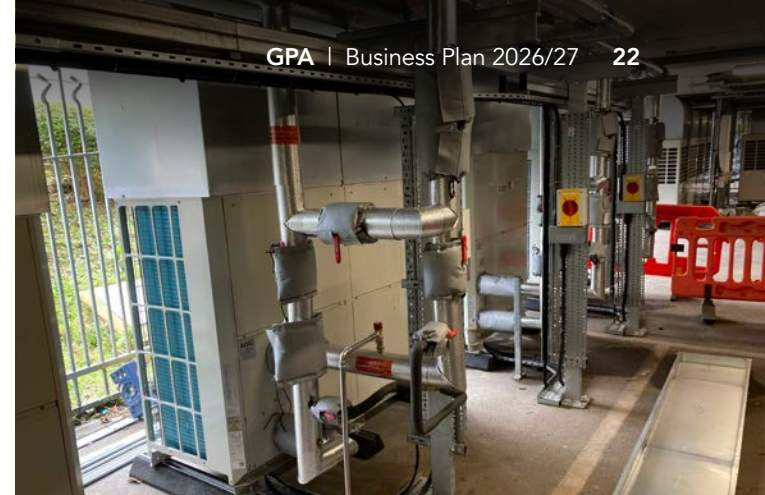
Air source heat pump at Coventry, Cheylesmore House.
